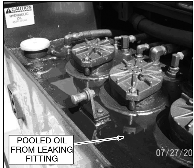
Leaking Hoses or Connections
