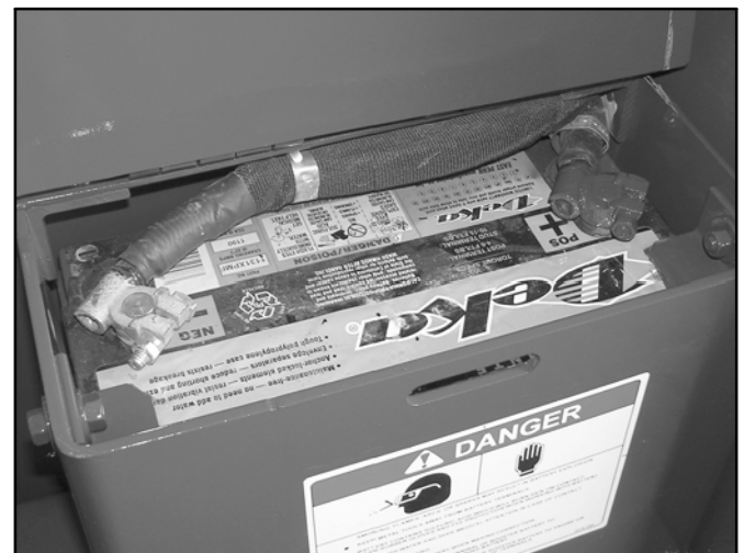
Battery Cable Properly Covered
