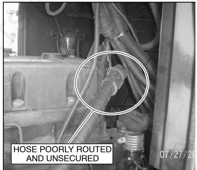
Improper Routing of Hydraulic Hoses or Improperly Secured Hoses
