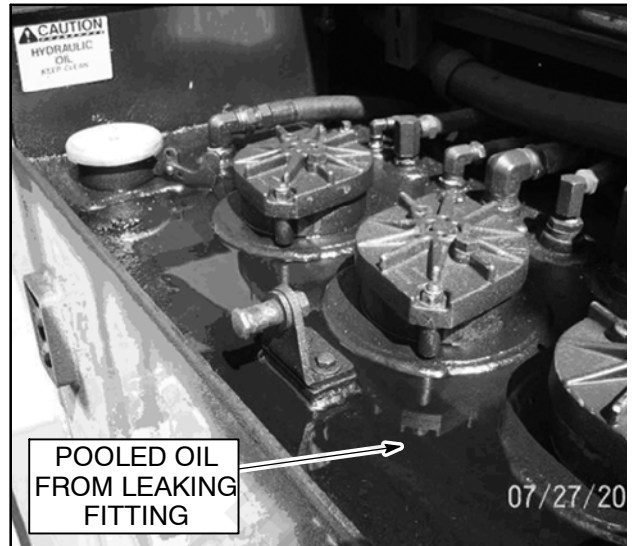
Leaking Hoses or Connections
