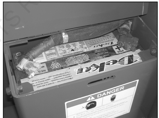
Battery Cable Properly Covered
